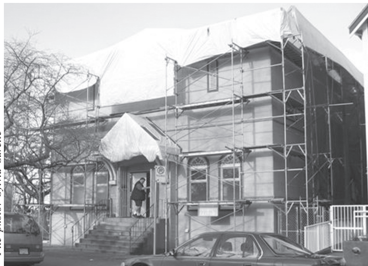
This is how the Ukrainian Cultural Centre in Vancouver looked in February, before the renovations were completed. Now, the scaffolds are gone, but a debt remains.
